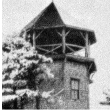
(TOP) Fig. 89: Original belvedere with log posts and railings.. (MIDDLE) Fig. 90: Rebuilt belvedere with 4x4 pressure treated wood members. (BOTTOM) Fig. 91: Front verandah showing log railings.
